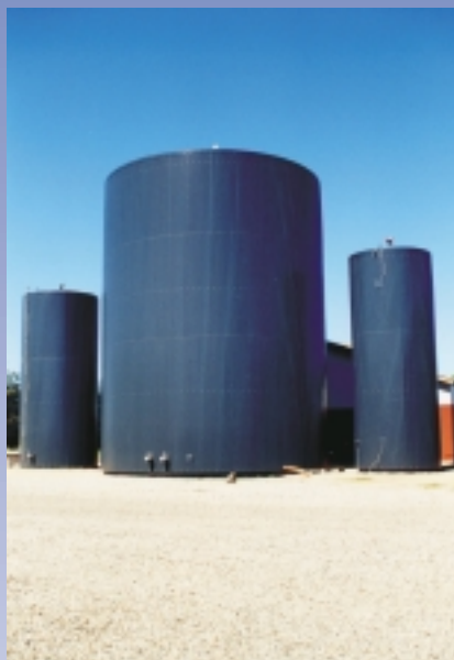
Smedemester farm biogas plant at Hemmet. The plant has a reactor of 800 m 3 and a 400 kW dual-fuel engine.
