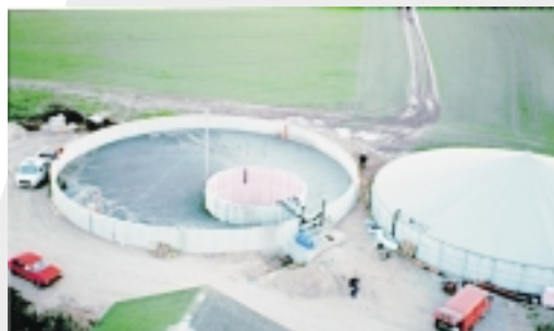
Low cost biogas plants with soft-top and integrated process tank
