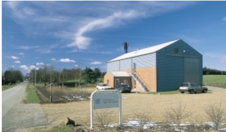
The gasification plant at Høgild, which has been running since 1994. The plant is currently being converted to use ordinary wood chips as fuel.
