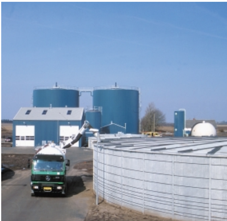
Several centralised biogas plants - like this one at Studsgård near Herning - process organic household waste at a price of DKK 40-50 per tonne.
