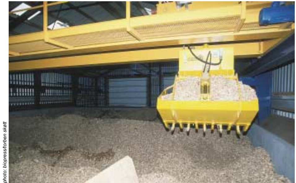
Wood chip storage with crane for the feeding of the wood chip boiler furnace at Harboøre. The crane can be automatically controlled and monitored from a screened control room.
